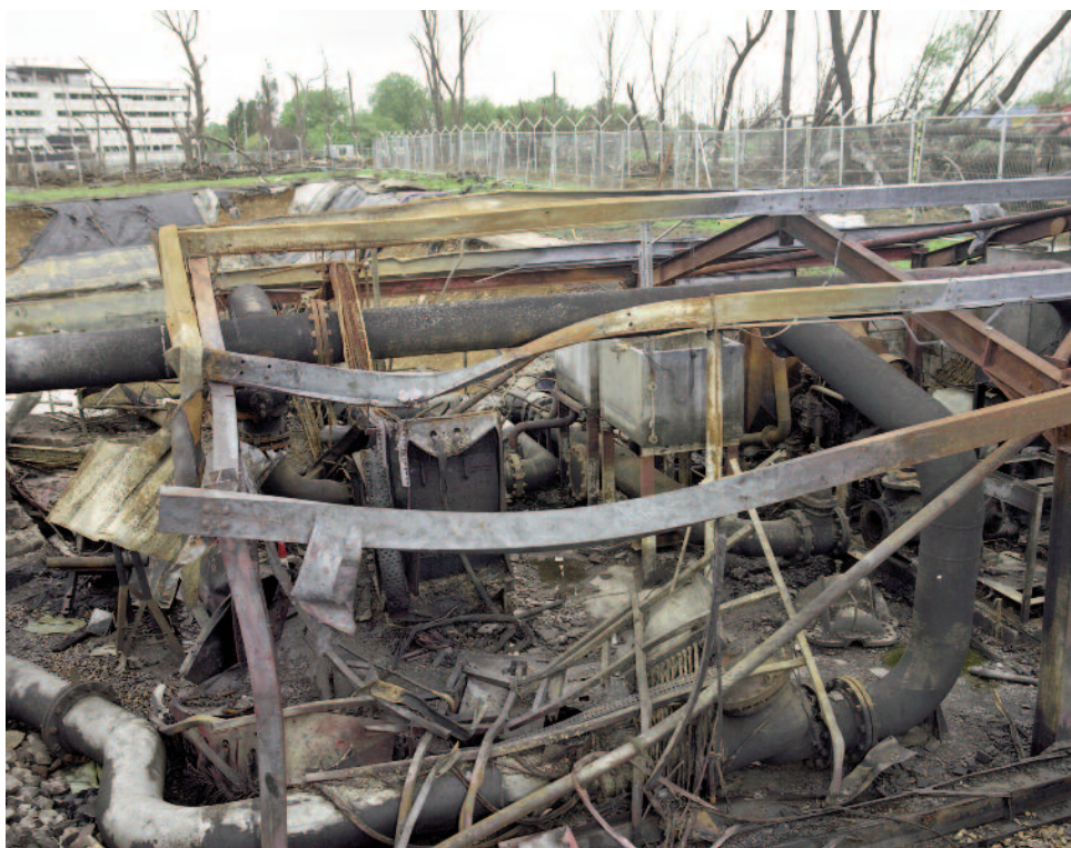
Figure 23 The remains of the fire pump house at the HOSL West site. The wall of bund A is approximately 5 m in front of this picture. The pump house is a prime candidate ignition source for the explosion at Buncefield
